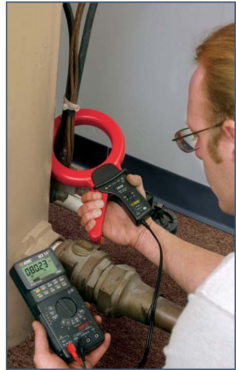
Model 2620 checking for ground fault currents
